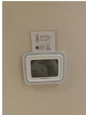
Guest room energy management
